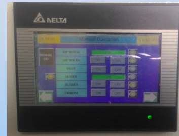
HMI with PLC (Full Touch)
